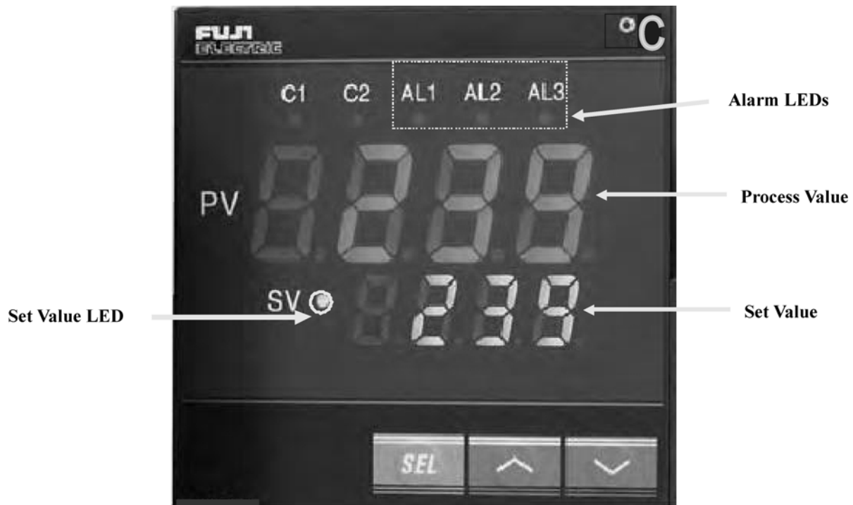
Figure 4-6. M501-TRS Temperature Controller Startup
